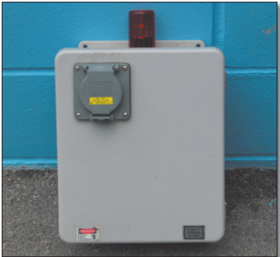
Figure 1. Electrical Control Panel With Generator Receptacle
