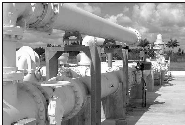
ASR Well No. 1 at the Miami-Dade Water and Sewer Department's West Wellfield.
