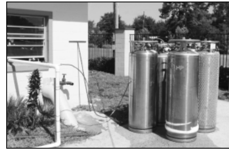
Figure 2: Piping for CO 2 Injection at Well 1. White PVC pipe provides water supply for CO 2 feed. Injection was done through pump column. Pump installed at a depth of 150 feet. CO 2 shown in 400-pound cylinders.
