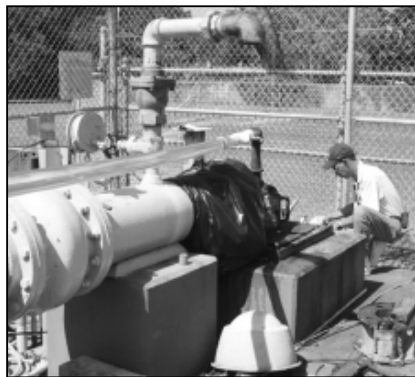
Figure 1: Wellhead piping at Well 3 for CO 2 injection. Note horizontal run of clear PVC connecting to 2-1/2 vertical steel tremie pipe. Injection was done through the tremie pipe terminating at a depth of 1,000 feet.
