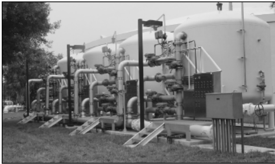
The dual media filters, together with chemical pre-treatment, are the key elements for arsenic removal, as well as removal of iron and other particulates from raw water.
