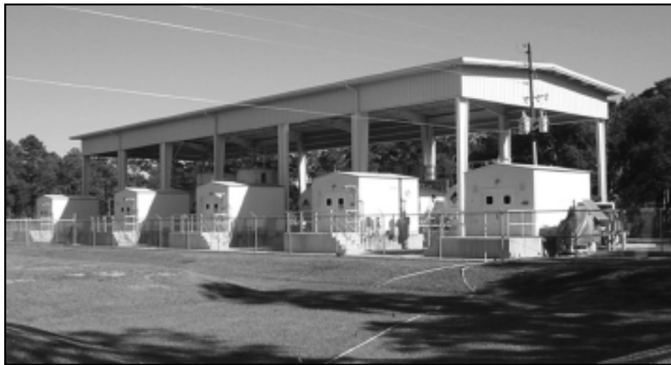
FIGURE 1: Interim Chemical Feed Facility used for regional blended water treatment.
