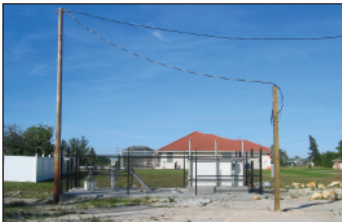
Figure 7 – New Southwest Supply Well
