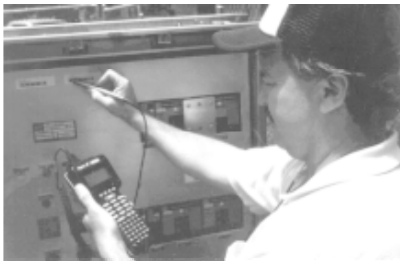
The author using a bar code reader at a remote lift station.
