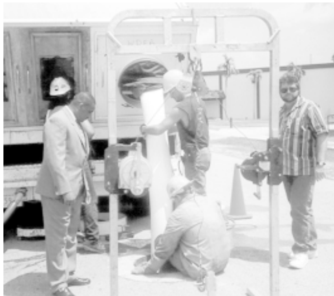
Public Services Director Kelvin Baker (left), Wastewater Division Manager William Rothman, and the Miller crew installing an eight-inch liner.
