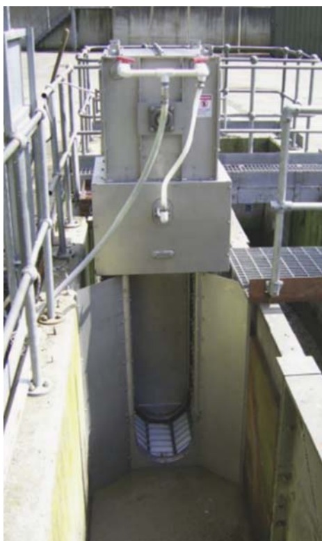
Figure 1. Center flow fine band screen installed in headworks channel.
