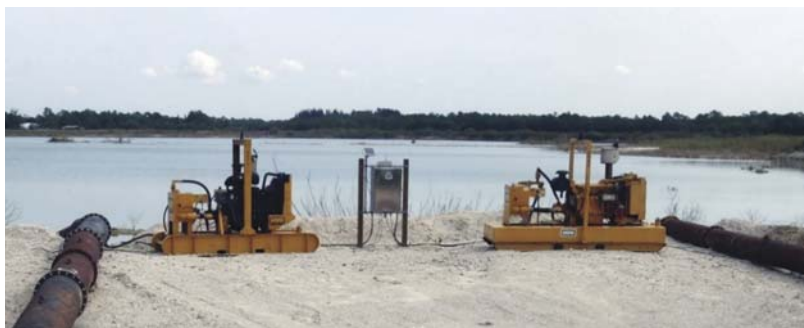
Figure 2. Pumps at the Southwest Aggregates withdrawal lake.
