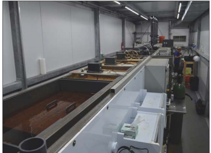
Figure 3. Flocculation-sedimentation was used as a pretreatment step for the Ozone-BAF system. Shown is the sedimentation basin, along with the chemical storage metering pumps and operator interface panels.
