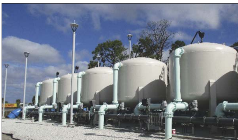
Figure 2. Water Treatment Plant No. 8 Anion Exchange Vessels
