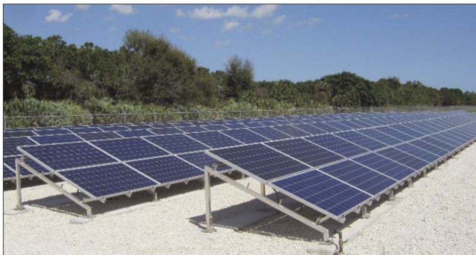
Figure 5. Southern Region Water Reclamation Facility Solar Panels
