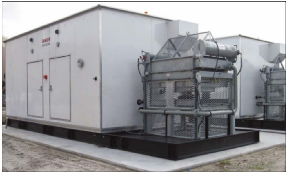
Figure 4. Southern Region Water Reclamation Facility Biogas Generator Enclosure
