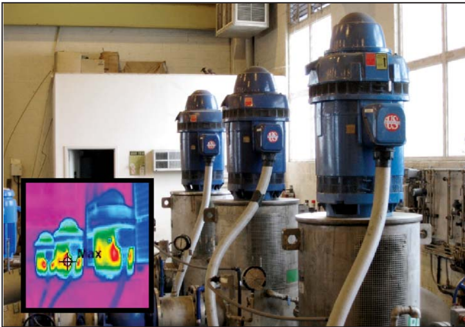
Figure 1. Pump Motors and Operating Temperature Gradient
