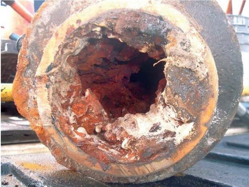
Figure 1. Sample picture showing renewal and replacement needs.
