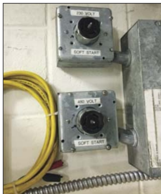
Figure 3. Power Cable Receptacles
