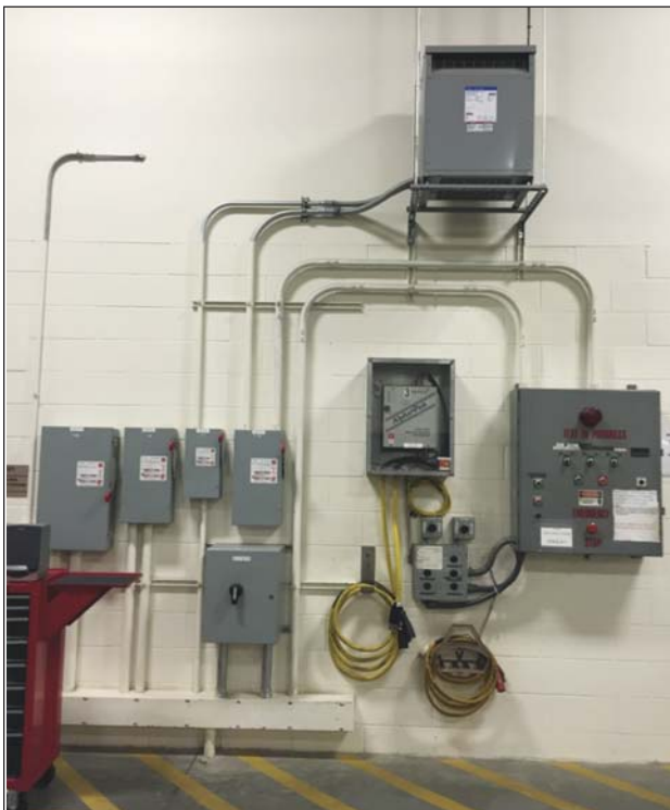
Figure 1. Pump Motor Test Panel
