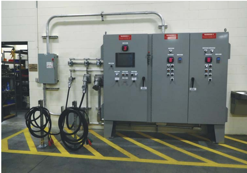
Figure 11. New Pump Motor Test Stand, Final Installation
