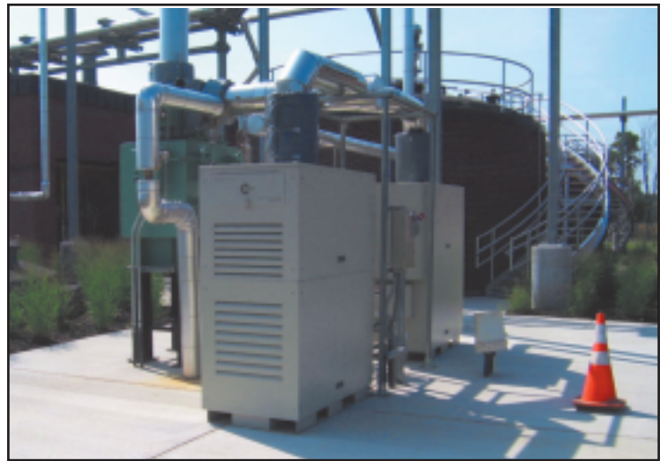
Thirty-kilowatt microturbines and gas-to-water heat exchanger.
