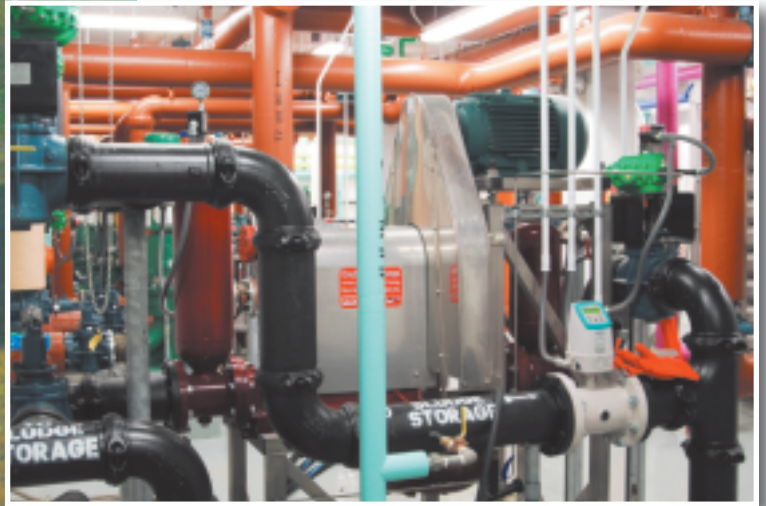
Above: Basement location of sludge pumps and heat exchangers. Left: An aerial view of the completed IBES.
