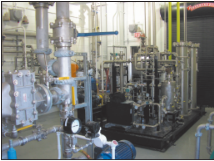
Digester gas room, microturbine gas compression, and scrubbing skid.
