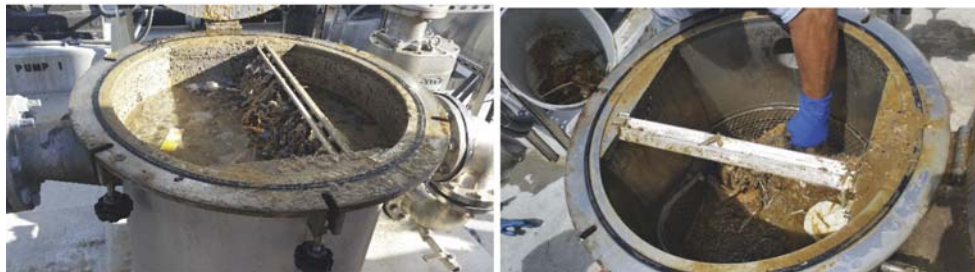
Figure 8. Basket Strainer Before (left) and After (right) Hot Water Flushing
