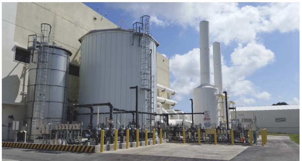
Figure 2. Fats, Oil, and Grease Receiving Station at the North Regional Wastewater Treatment Plant
