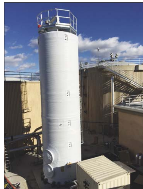
Figure 6. BiogasClean biological H 2 S removal system at the Truckee Meadows Wastewater Treatment Plant in Reno, Nev.
