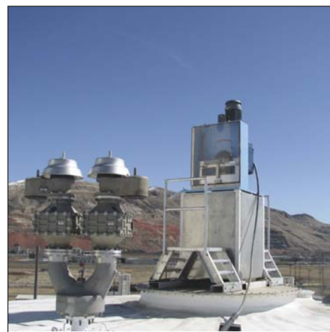
Figure 2. Linear motion mixer for sludge mixing on a 95-ft-diameter steel floating digester cover at the Salt Lake City Water Reclamation Facility.
