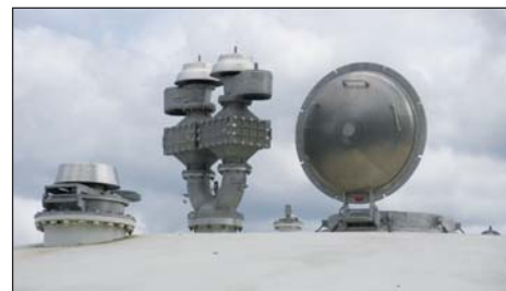
Figure 10. Digester cover with 48-in. manhole cover, redundant PRV/flame arrester with three-way safety selector valve, and secondary pressure relief via the emergency pressure relief manhole cover.
