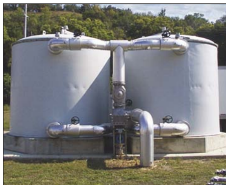
Figure 5. Fiberglass-insulated vessel with Iron sponge media at the Sioux City (Iowa) Wastewater Treatment Plant.
