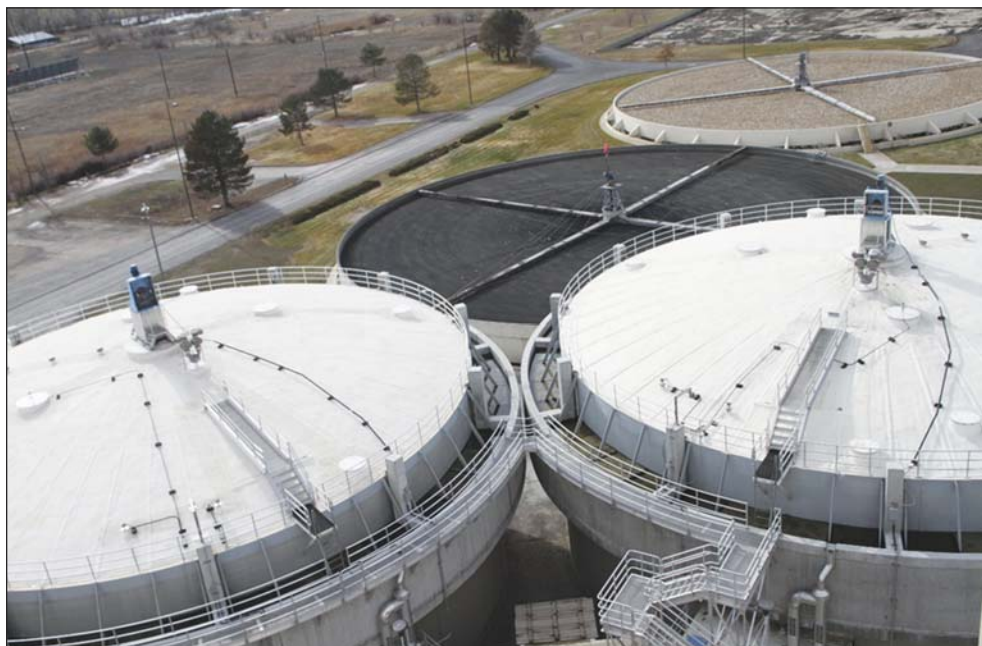
Figure 1. 95-ft-diameter steel floating covers at the Salt Lake City Water Reclamation Facility.
