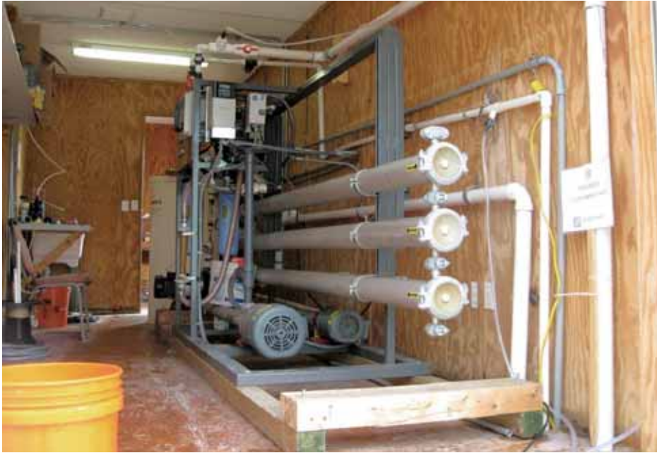
Figure 3. Osmonics Reverse Osmosis Skid 2:1 Configuration
