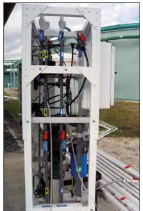
Figure 2. Florida Atlantic University Reverse Osmosis Skid
