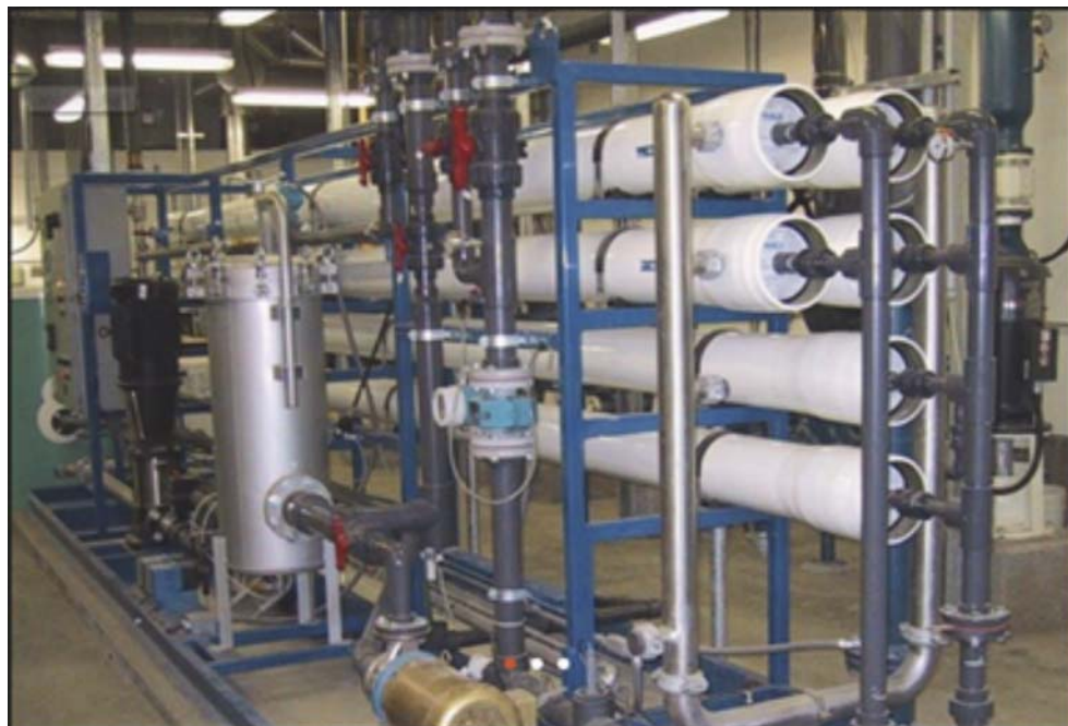
Nanofiltration pilot plant.
