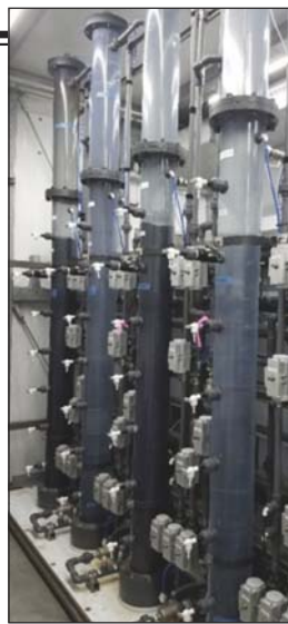
Figure 6. Biologically Active Filters
