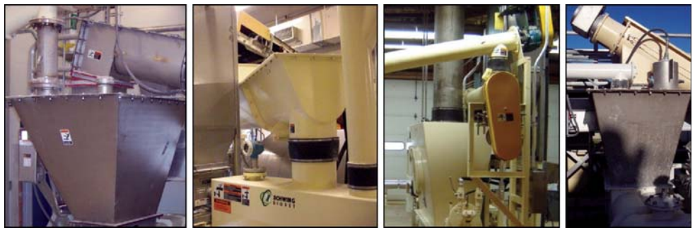
Figure 3. Equipment Showing Connections in Hopper
