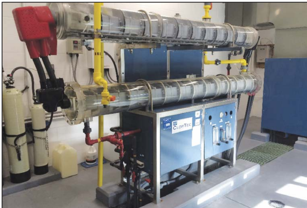
Figure 10. Old Onsite Sodium Hypochlorite Generators at Lake Park Water Treatment Plant
