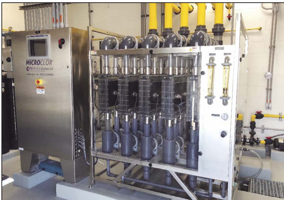
Figure 11. New 2000-ppd Onsite Sodium Hypochlorite Generators at Lake Park Water Treatment Plant
