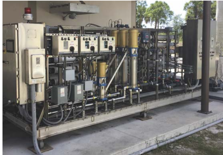
Figure 4. Pilot Unit Pumping and Power
