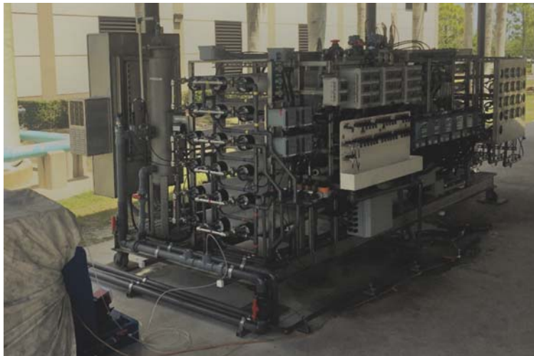
Figure 3. Pilot Unit Instrumentation
