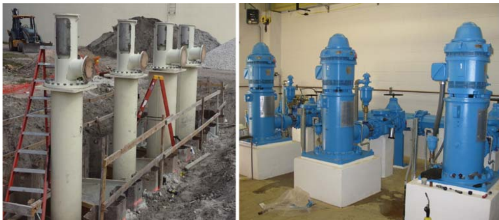
Figure 2. Installation of vertical turbine pumps in barrels; motors have not yet been installed.
