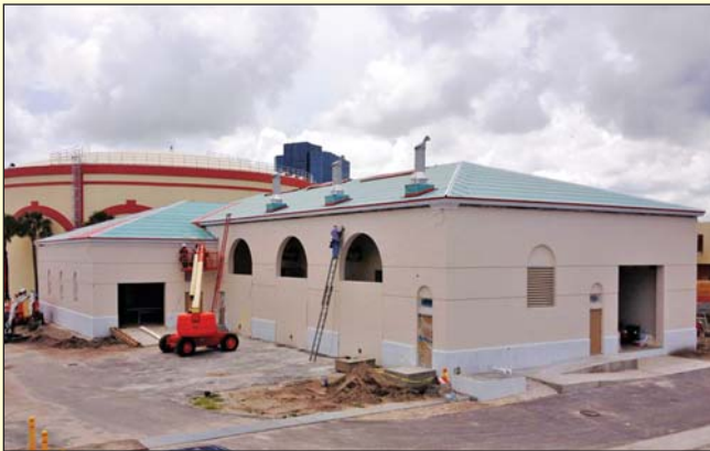
Figure 4A. New Electrical/Generator Building Increases Reliability of WTP Service.
