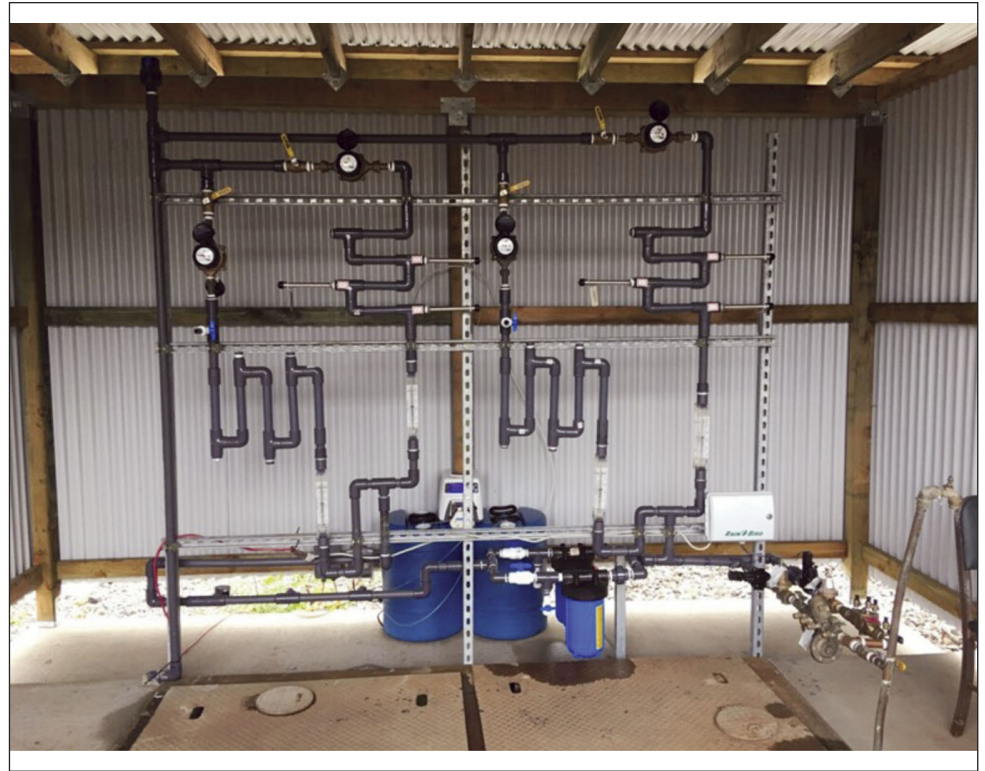
Figure 1. Corrosion Loop Test Rack Design Example (Maui, Hawaii) (photo: Angela Rodriguez)
