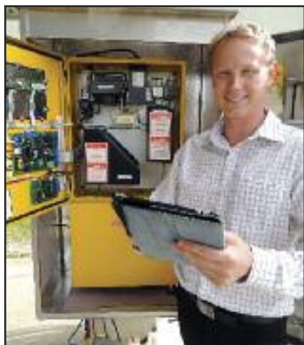
Albert Bock performs a system check on the digester nutrient analyzer system.
