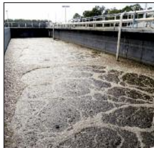
The facility's digester during the aeration cycle performing ammonium and phosphorus reduction.
