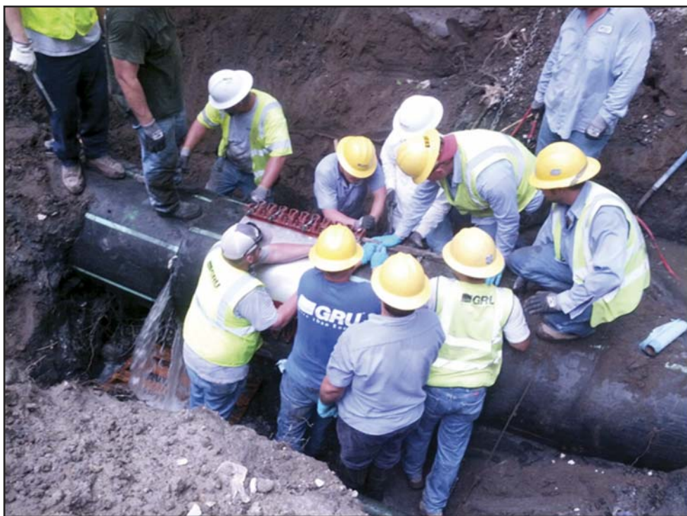
Figure 2. Highly visible wastewater collection system failure requiring a major emergency response.
