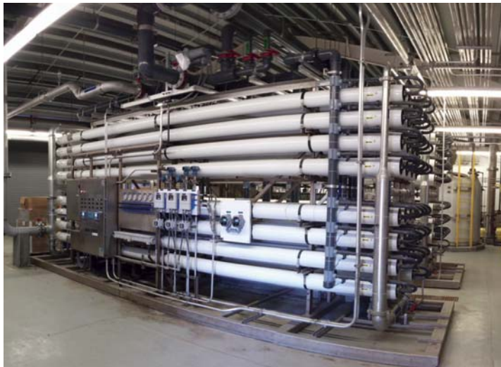
The modified and expanded reverse osmosis skids.
