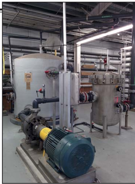
The then-new membrane feed pumps.
