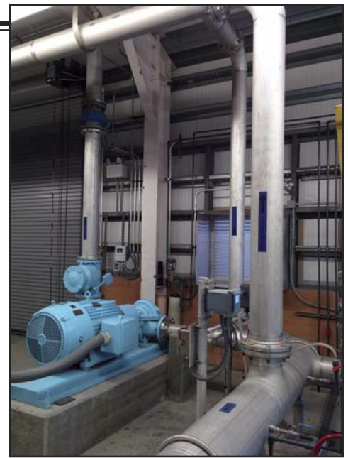
The new reverse osmosis cleaning pump.
