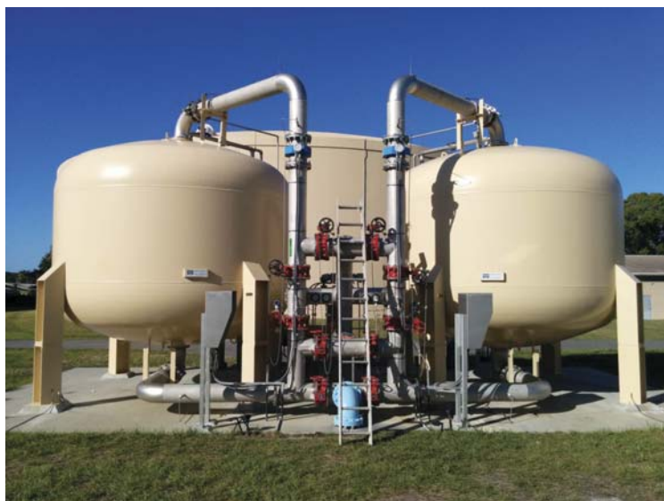
The reverse osmosis water treatment plant No. 1 arsenic adsorption system.
