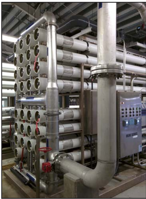
The feed, with expanded stainless manifolds, on the reverse osmosis skids.
