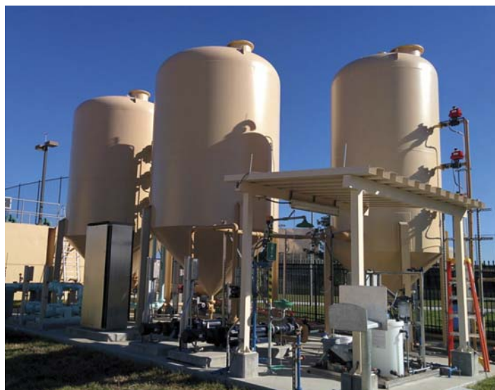
The reverse osmosis water treatment plant No. 1 decant and residual holding system.
