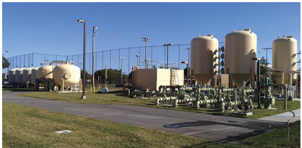
From left to right: the four existing dual media filters, the arsenic adsorbers, the backwash holding tank, the booster pumps, and decant system.
