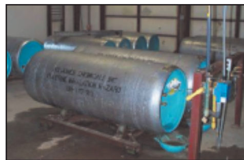
High Consequence Asset Susceptible to Multiple Hazards
